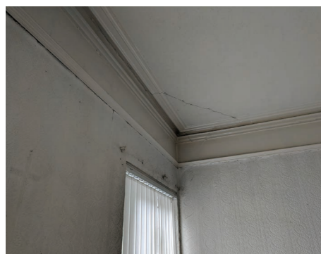
Cracking to the outer corner of the building showing some previous structural movement
