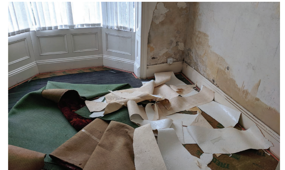
Damp caused by the external rainwater pipe and gully
