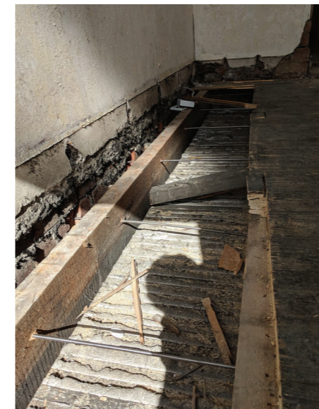
The tie rods shown after installation through the gable wall and joists
