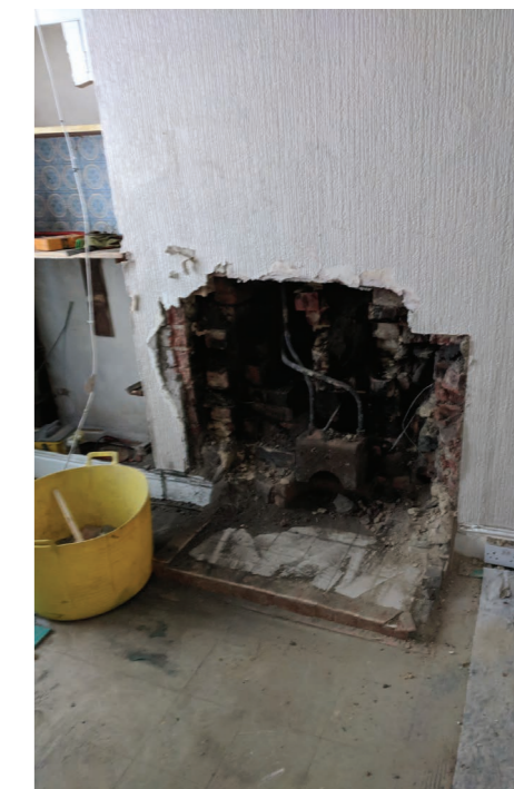
Rear chimney breast prior to its removal, showing the old back boiler
