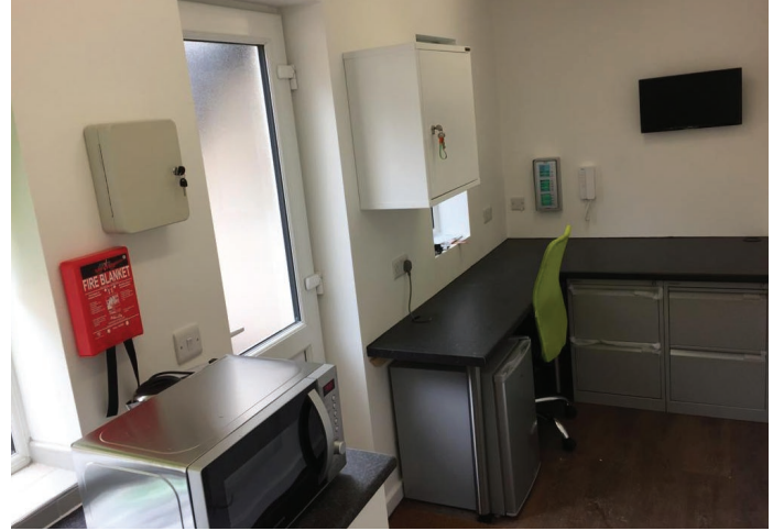
Care workers' facility and office installed with CCTV monitoring, incoming data lines and control points for the fire alarm and intercom system
