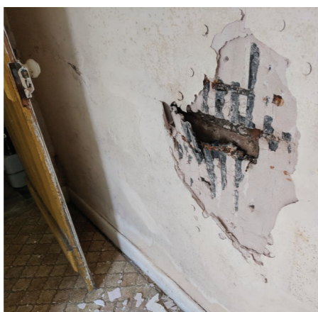
Failing existing tanking solution to the kitchen area
