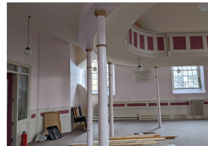
Another shot of the underside of the balcony showing the non-original paneling to the front
